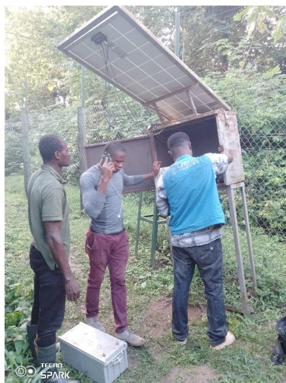
Checking the solar panels
